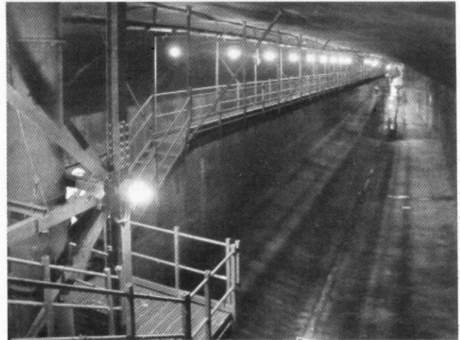
View back towards the access tunnel from the gantry above the pump shaft. Luckily the chamber was empty, otherwise the visit could not have taken place. Photo Clive Penfold
